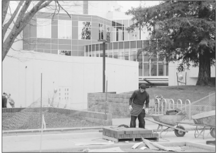
ROAD CLOSURE – Landscaping and other improvements on the east side of the University Union are expected to be completed this spring. Instead of a busy road, the area will feature shaded lawn and sidewalks, and the grassy area at the outdoor stage will be extended.
