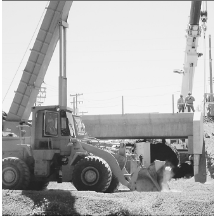
DIG IN – Work continues on the new bicycle and pedestrian underpass on the west side of campus, which will provide access to the University from 65th Street. The $2.5 million project is funded through federal transportation and air quality programs.
