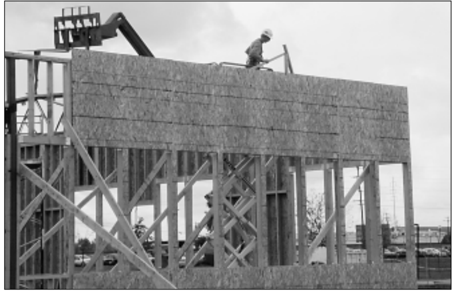
GOING UP – Work continued over winter break on the Steven Lee Yamshon Alumni Center. It will house the CSUS Alumni Association, which is celebrating the 50 th anniversary of its founding this year. The center is due to be completed by early summer, in time to host special events during the upcoming 2000 U.S. Olympic Track and Field Trials at Hornet Stadium. Yamshon, a CSUS alumnus, donated $1 million to help build the $2.2 million, privately funded facility.
