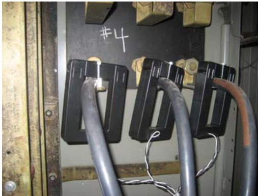
Figure 3. Main Transformer Current Transducers
